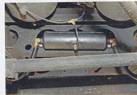
9. Here's the completed front suspension upgrade. As the air bag compresses, the air escapes through the larger line and into the ping tank, resulting in softer compression characteristics and a smoother ride. Air line routing from the compressor to the tank depends on the particular motorhome, but is usually handled with
